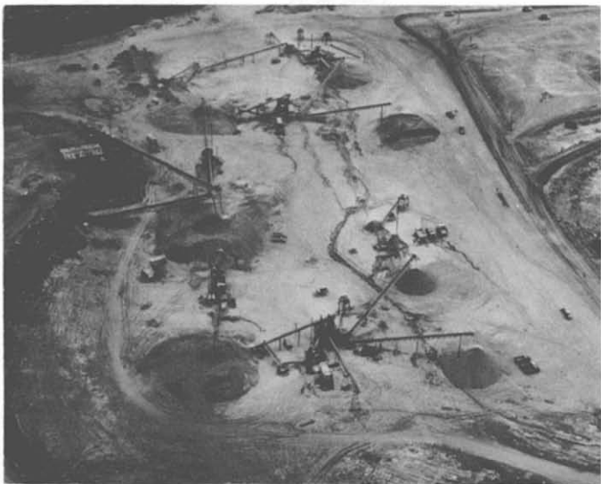
37. University Quarry—Saigon. This site derived its name from the fact that it was near the future Saigon University. In February 1966, a few months after its opening, the quarry had a 250 tons-per-hour crushing plant in operation, making rock for use throughout the greater Saigon area. In November 1966, a 400 ton-per-hour crusher was added and aggregate production jumped to an average of 6,500 tons per day. In January 1967, a hot-mix asphalt and concrete batch plant were set up. The new diversity of products led to the imposing new site title: "Saigon University Materials Products Company" or, for short: SUMPCO.
