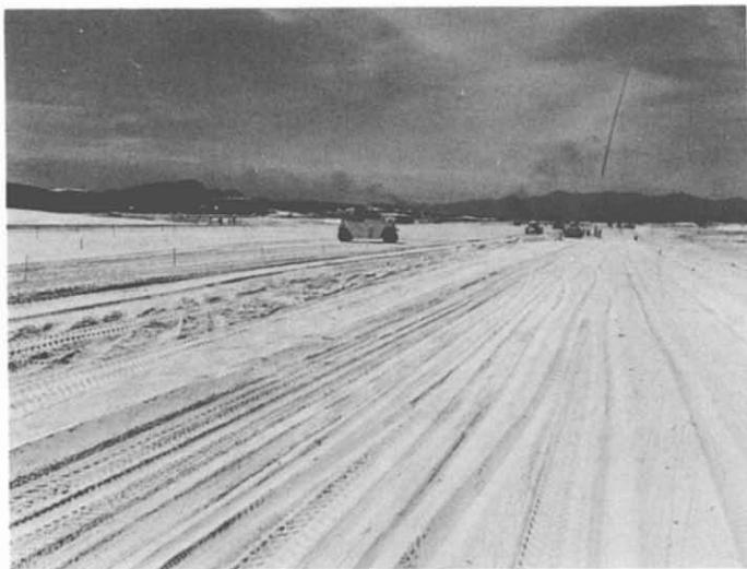
21. Cam Ranh Airfield—Site Preparation. Photograph shows the prevalent sandy character of the Cam Ranh peninsula. The site is being prepared for a 10,000' expeditionary runway and taxiway. A critical factor during construction was the attainment of sand compaction to successfully support the runway/taxiway and to be able to withstand the repeated aircraft landings. Based on extensive tests, the critical problem was resolved by flooding the area for 24 hours and then compacting with a vibrator compactor.
