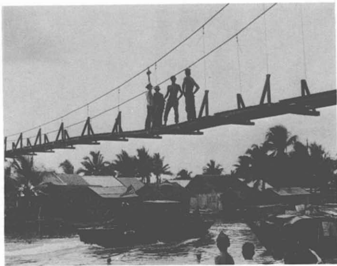
76. Suspension Bridge—Thu Thua. Construction of this suspension bridge was started by Seabees from Seabee Team 0604 (NMCB-6). This 50-meter footbridge was then completed by Team 0410.
