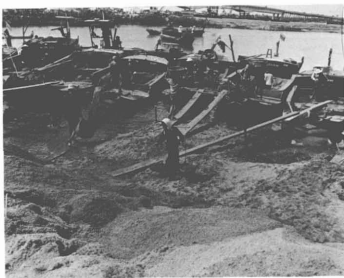
18. Newport (Saigon)—In Construction. Since the Saigon River bottom was silt, dredged fill from the river could not be used and fill had to be brought in from other areas. Sand was brought in at the rate of 7,000 cubic meters a day; and, unbelievably, about 3,000 cubic meters of this was delivered by sampans.
