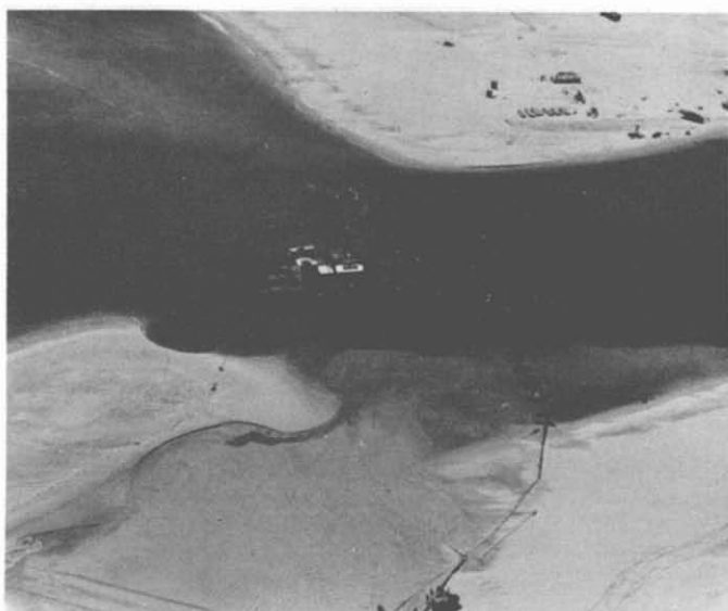
33. Pipeline Dredge: SEABEE I. The 20-inch pipeline dredge SEABEE I is clearing the entrance channel to the Han Giang River, at Cua Viet.
