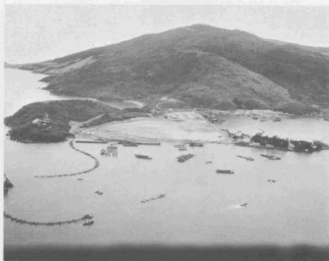
1. Observation Point (Da Nang) Port Facility—July 1966. Work involved dredging an entrance channel and turning basin to a depth of 39 feet; the bulk of the dredged material was used to fill a 45 acre tidal swamp, thereby creating a staging area for off-loaded supplies. A 2,000 sheet piling bulkhead (seawall) was built. Two jacket-type piers were to be installed. Each pier is 90' \times 600' . These piers were prefabricated at Poro Point, Philippines, by RMK-BRJ and shipped by barge to Da Nang. The abutment for a third pier, a mobile DeLong type, was also in the job.
