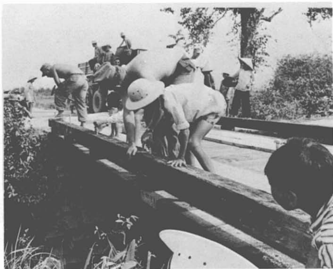
77. Replacing Collapsed Bridge—Phuong Dien. A "Civic Action Team" from NMCB-10 and local Vietnamese work together to complete a new bridge near Phuong Dien, replacing old, collapsed structure.
