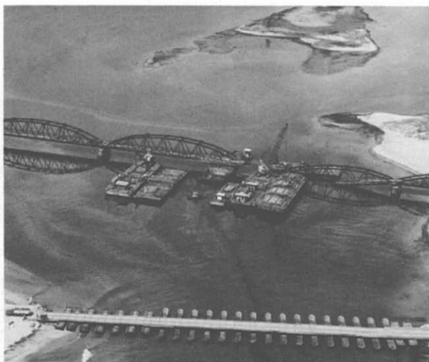
54. Nam-O Bridge. The Nam-O Bridge is a combination railroad and highway bridge; it is located 10 miles north of Da Nang, on Route QL-1. It is a vital supply line to Phu Bai and the North. On the night of 13 April 1967, the Viet Cong mined and completely demolished one of the center piers, dropping the ends of two of the bridge's five 140' steel truss spans. The destroyed pier was replaced by a steel pile jacket pier. The affected spans were repaired as needed and reset in position. Note the interim use of the pontoon bridge.
