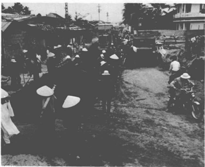
48. Street Repair—Quang Ngai City. Typical scene in the program of street and road upgrade/rehabilitation. This is Tran Hung Dao Street, in Quang Ngai City, in Military Region I.
