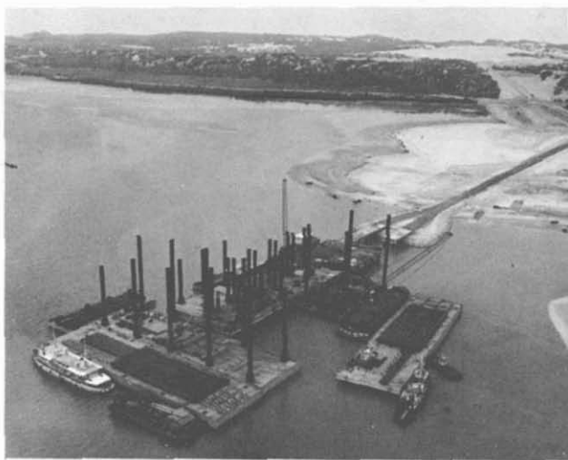
23. DeLong Pier—Cam Ranh Bay. The U.S. Army had procurement responsibility for the DeLong prefabricated pier—an “advanced base” type of pier—shown here in process of installation. The OICC/Contractor assisted in preparing sites for such installations—building bulkheads; providing dredge fill for causeways; supplying equipment and personnel as needed. DeLong piers were also installed at Da Nang and Qui Nhon.
