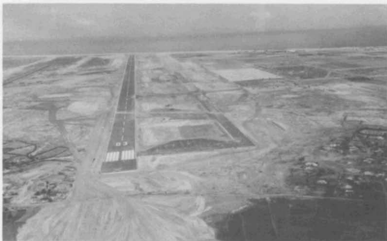
9. Tuy Hoa Airfield. In construction, November 1966. The Air Force received special authorization from OSD to build the Tuy Hoa Airbase. The facility was built under a "Turnkey" form of contract with Walter Kidde Constructors, Inc., at a cost of $52 million.
