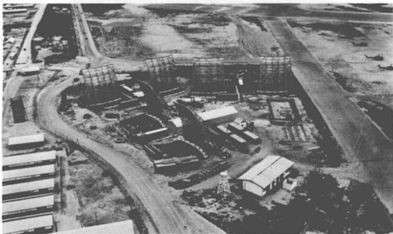
60. Communications Facility—Nha Trang. In June 1965, RMK began construction of antenna foundations and support buildings for this communications facility at Nha Trang; in July, construction was begun on barracks and messing facilities for U.S. Special Forces. The foundations were completed in July 1965; the cantonment, in January 1966. The electronic phases of the installation were accomplished by Page Communications. Nha Trang was a terminal for voice submarine cable from the Philippines, and a link in a tropospheric scatter radio system.
