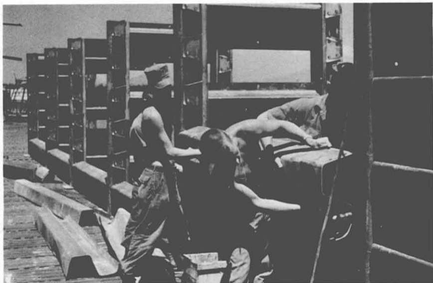
87. Aircraft Revetment Assembly—Phu Bai. Seabees of NMCB-133 assemble revetments on the aircraft parking apron, at Phu Bai, for Marine Air Group 36 (MAG-36). The revetments are built in a "U" to envelop the aircraft on three sides. The assembled revetments are filled with sand.
