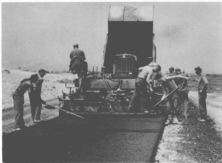
90. Road Rehabilitation—Vinh Dai. Members of NMCB-53 pave a road with asphalt, at Vinh Dai. Original road surface had to be totally reconstructed.
