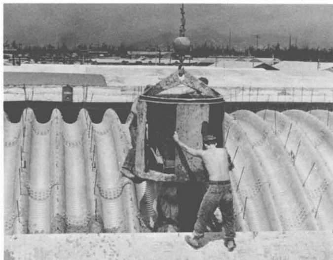
75. Wonder Arch Aircraft Shelter—Military Region I. Sea bees of NMCB-121 pour concrete to form a protective cover for a "Wonder Arch" aircraft shelter for Marine Aircraft Group 16, located in Military Region I.
