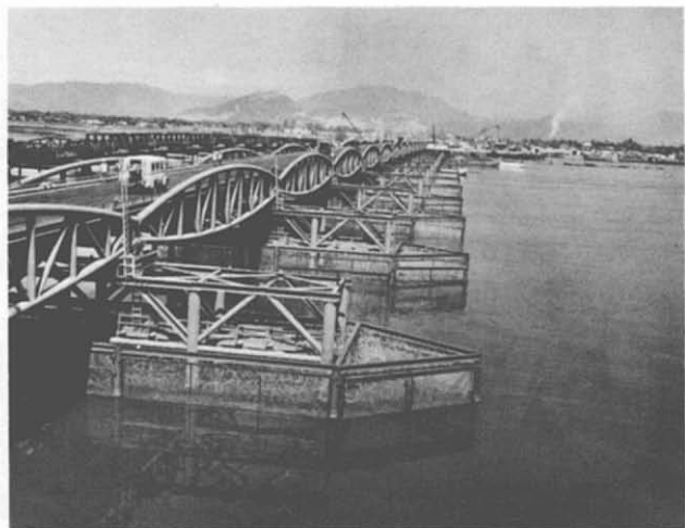
52. New Da Nang Bridge Detail. Bridge pier protection was undertaken as a deterrent to enemy attempts (by frogmen and floating charges) to destroy or damage the structure. Pier protection included pier lighting and approach lighting; steel bracing to pier structure for added support; and framing, chain link panels, and loosely-placed concertina wire.
