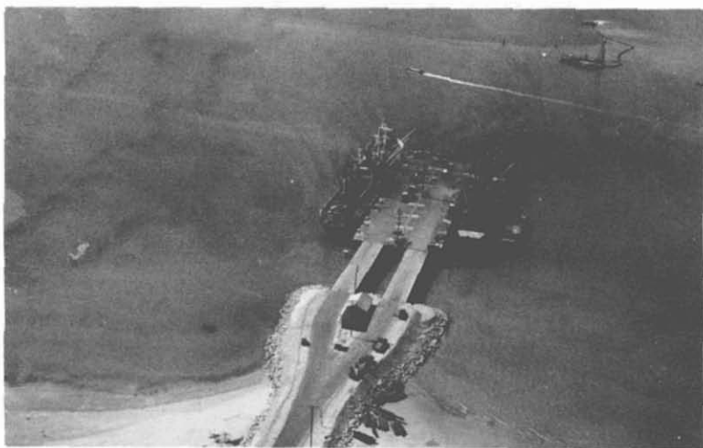
25. Ammo Pier at Cam Ranh Bay. Photo shows construction completed on the 3,600' earth causway. Installation is underway to form a DeLong deep-draft ammunition pier that will measure 450' long by 120' wide. The new facility will be capable of simultaneously handling two C-3 class freighters at its 2 berths.
