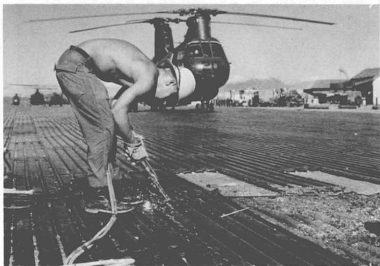
71. M8A1 Parking Apron Repairs—Dong Ha. Seabees of NMCB-11 repair and relay a type M8A1 steel matting of a parking apron which was damaged by enemy mortar fire.
