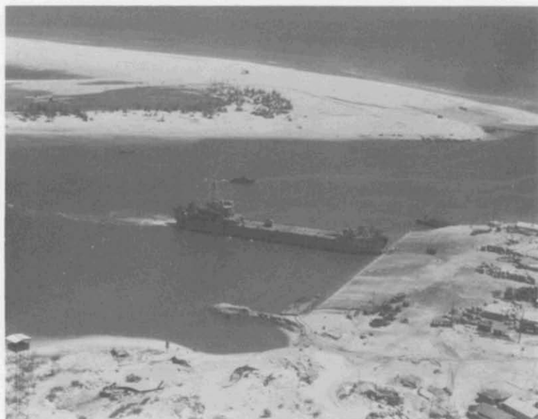
8. LST Ramp at Cua Viet. Cua Viet is a location about 6 miles from the DMZ. Urgently needed for military operations, this LST ramp had to be built under extremely hazardous dredging conditions (typhoons and heavy seas), and the prevalence of Viet Cong who were very active in the area.
